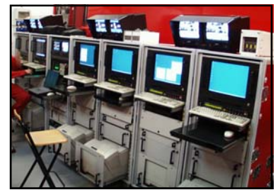
Quentor telemetry cabinets
